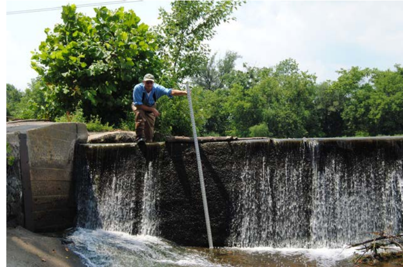
Photo 1 - Existing dam upstream of Wehr's Covered Bridge. Dam height is approximately 6-foot.
