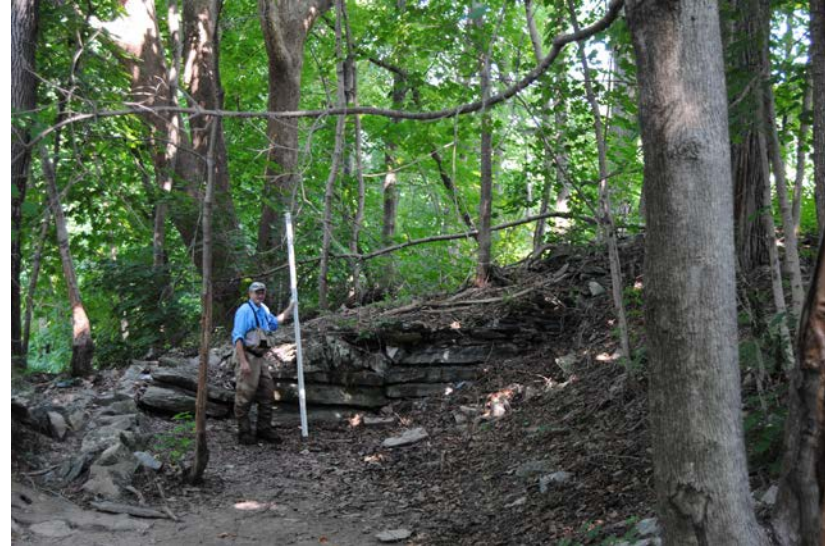
Photo 5 - Man-made berm which creates a “pinch point” along the creek which causes park flooding.
